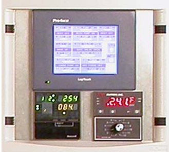
Front Control Panel
